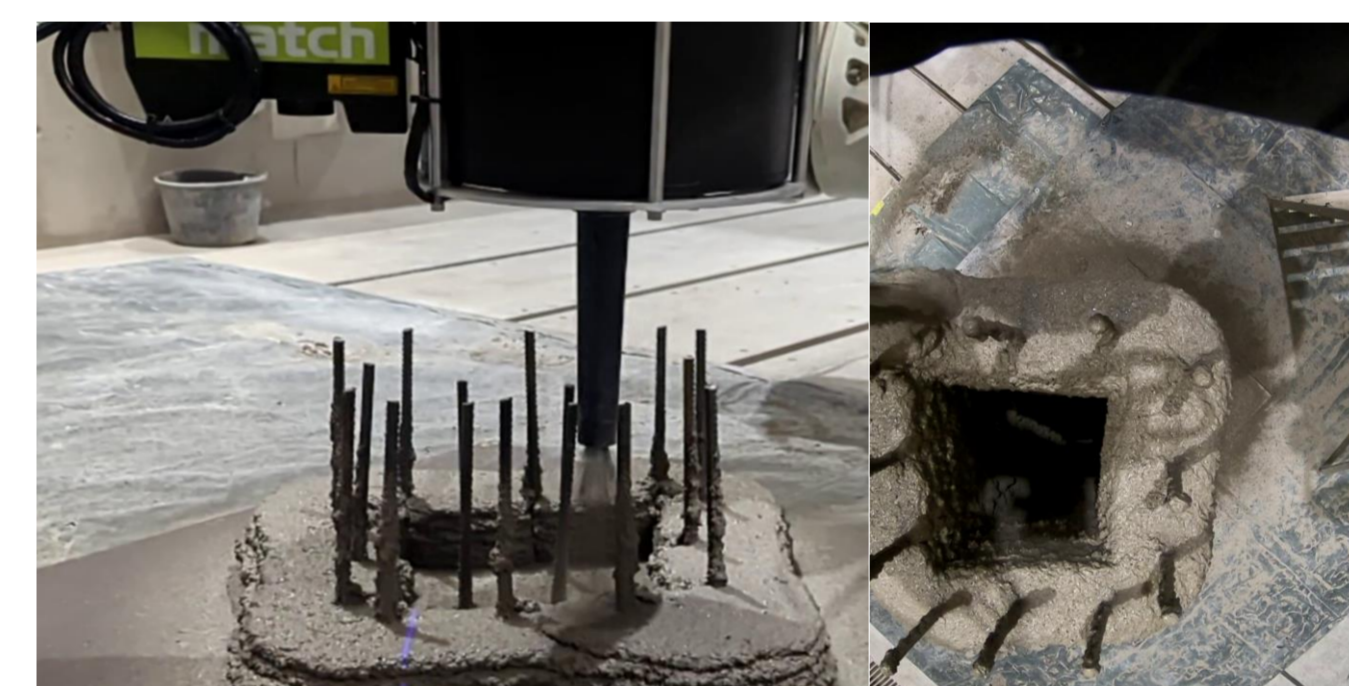
Fig. 5: The strand control is influenced by rebar. In-process image evaluation allows for object classification.
